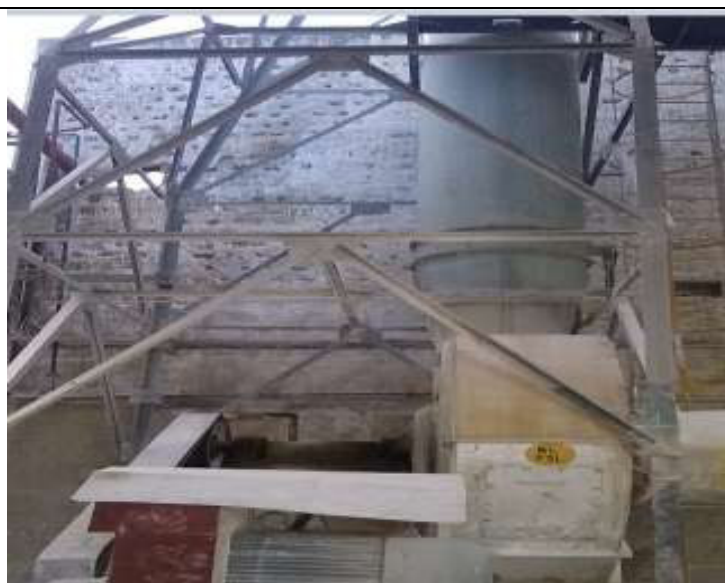
Bag filter _secondary Exhaust blower(NIRO III
