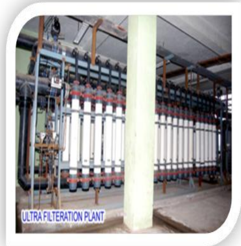
Ultra Filtration Plant
