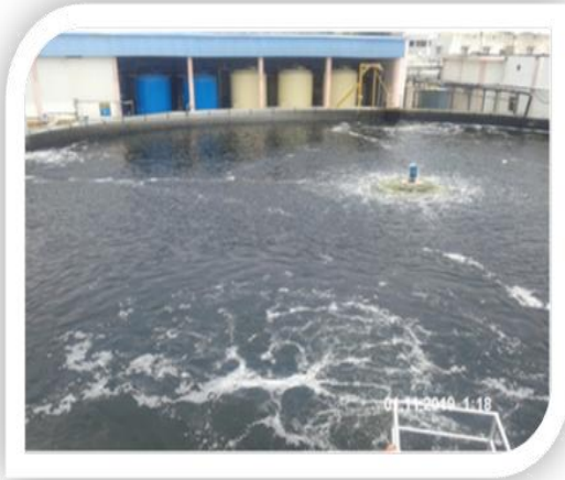
Collection cum Homogenization Tank
