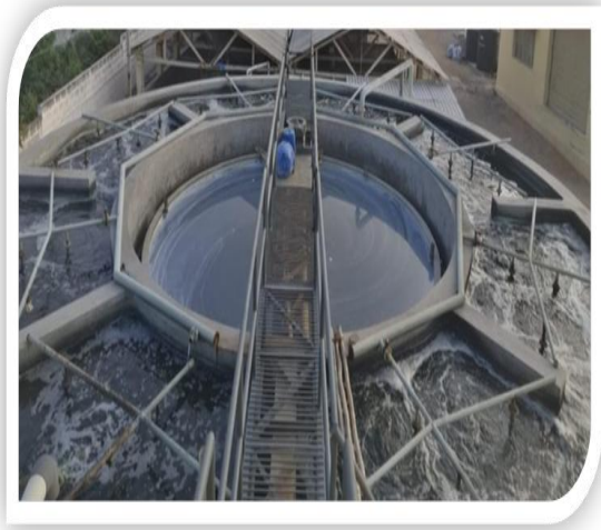
Aeration & secondary clarifier
