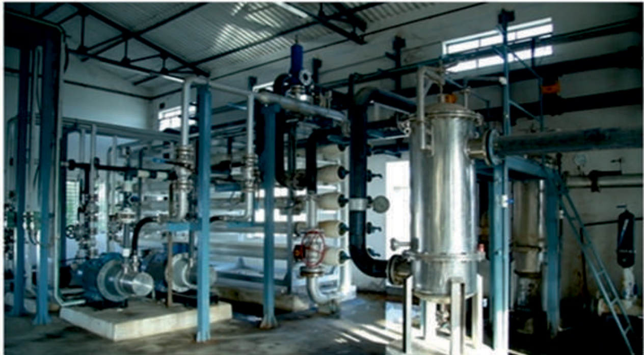
RO - Plant System
