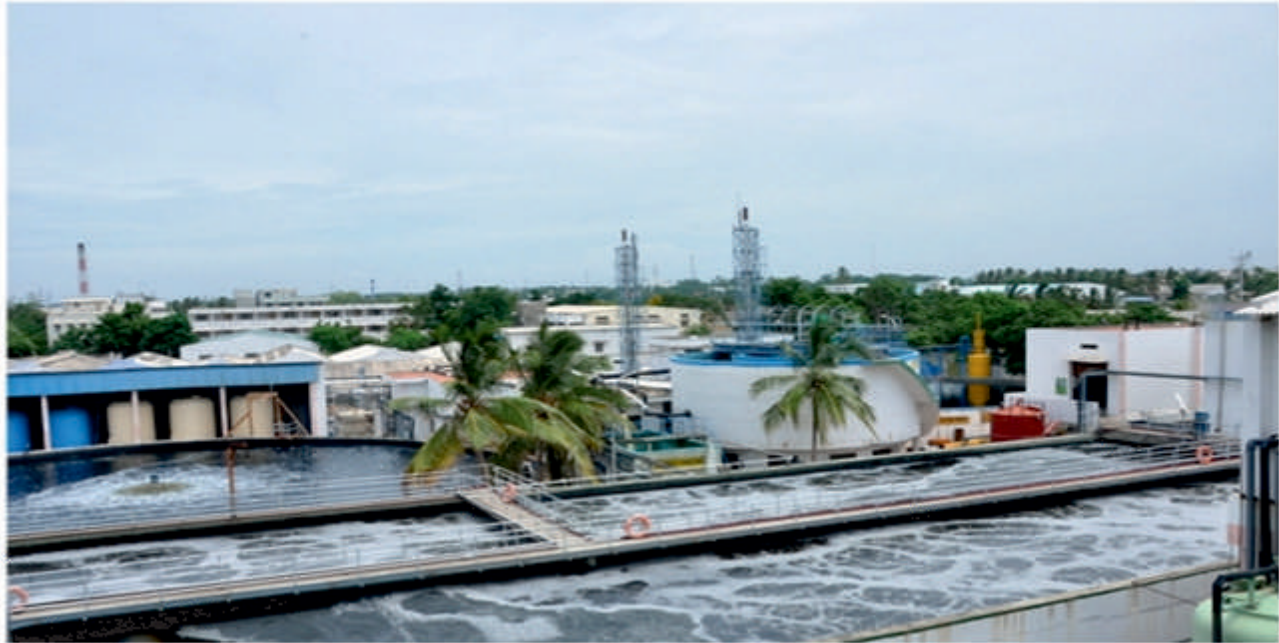
Effluent Treatment Tanks
