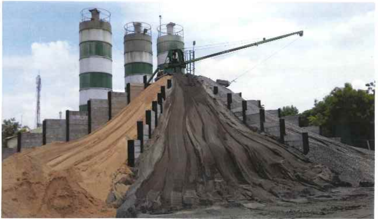
Ramp for Loading Fine Aggregates - 30 m 3 /hr Plant
