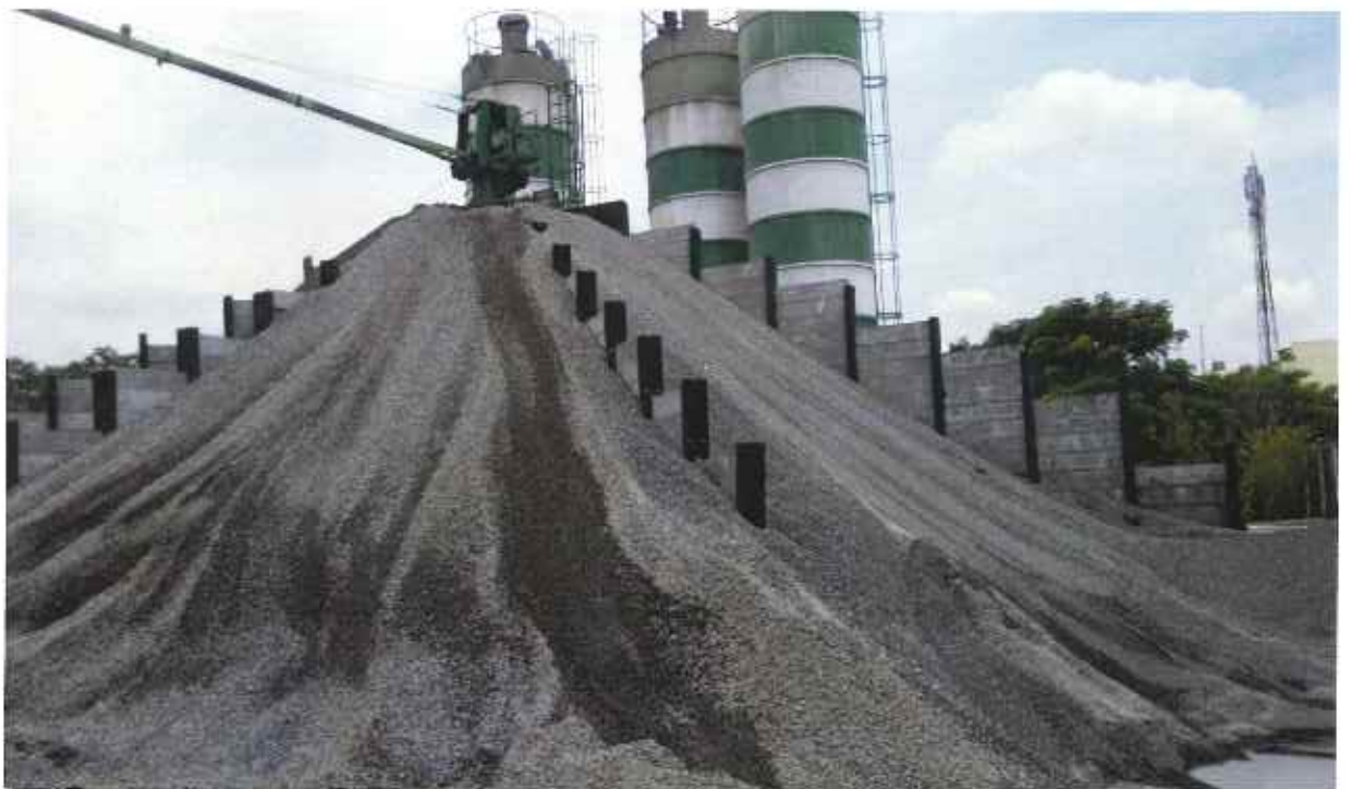
Ramp for Loading Coarse Aggregates - 30 m 3 /hr Plant
