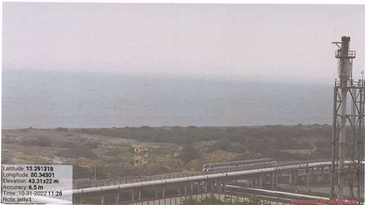
Fig.1 A view of pipeline from Indian Oil LNG Pvt Limited Jetty to the Storage unit
