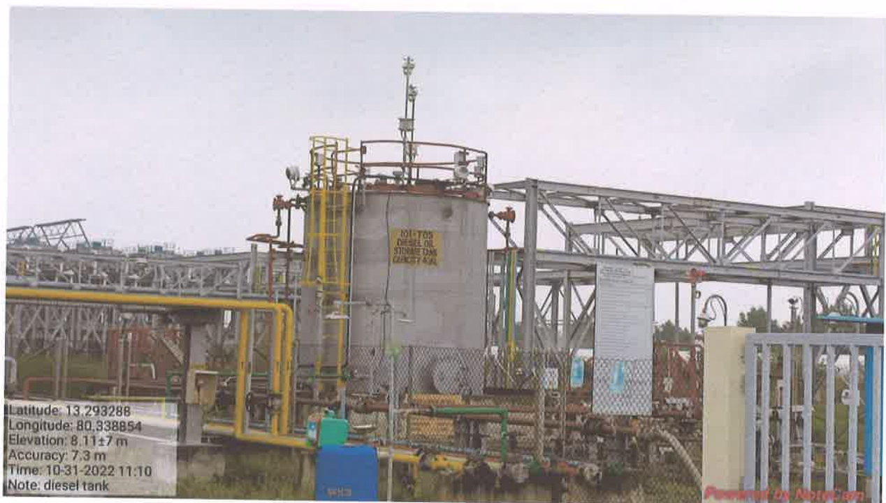
Fig.4. Diesel Oil Storage tank
