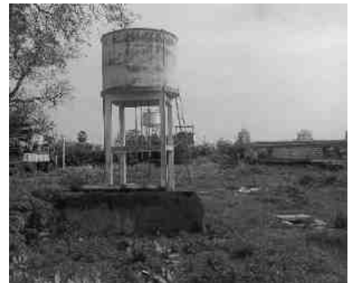
Water Tank, Alagulam
