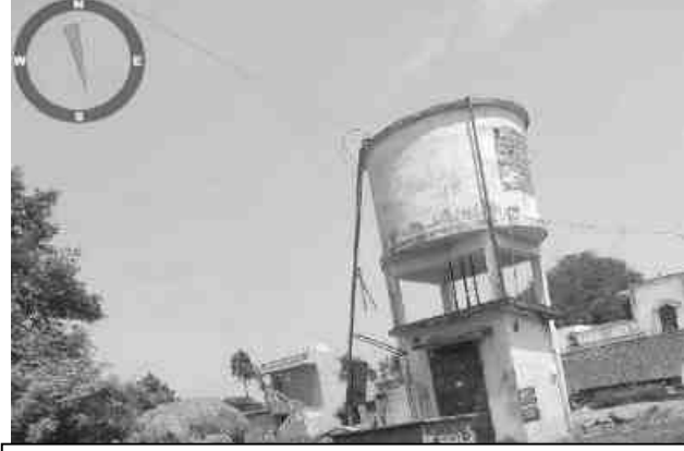
Menallur – Overhead Water tank
