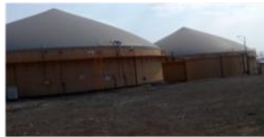
Digester (6600 cu.m/each (3 nos))
