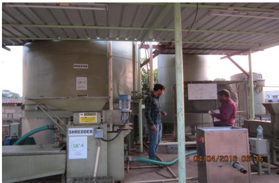
Gas Power System 1 MTD Plant In AOL, Bengaluru
