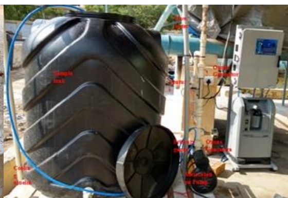
Fig.2 - Pilot plant ozonator
