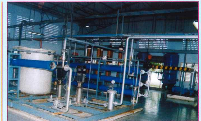
REVERSE OSMOSIS SYSTEM INSTALLED IN ONE OF THE INDIVIDUAL TANNERY
