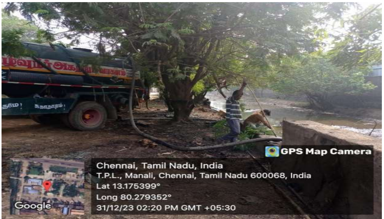
Cleared area along the canal near Indian Additives compound wall in CMDA Steel complex in Sathankadu.
