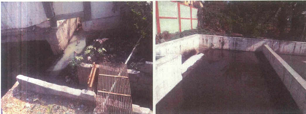
Vellakuttai STP (diversion of sewage from drain)
