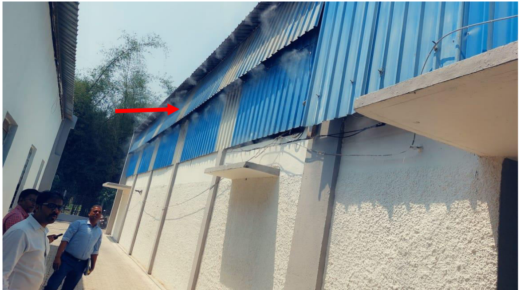
Mist filtration provided at Industrial louvers of unit shed
