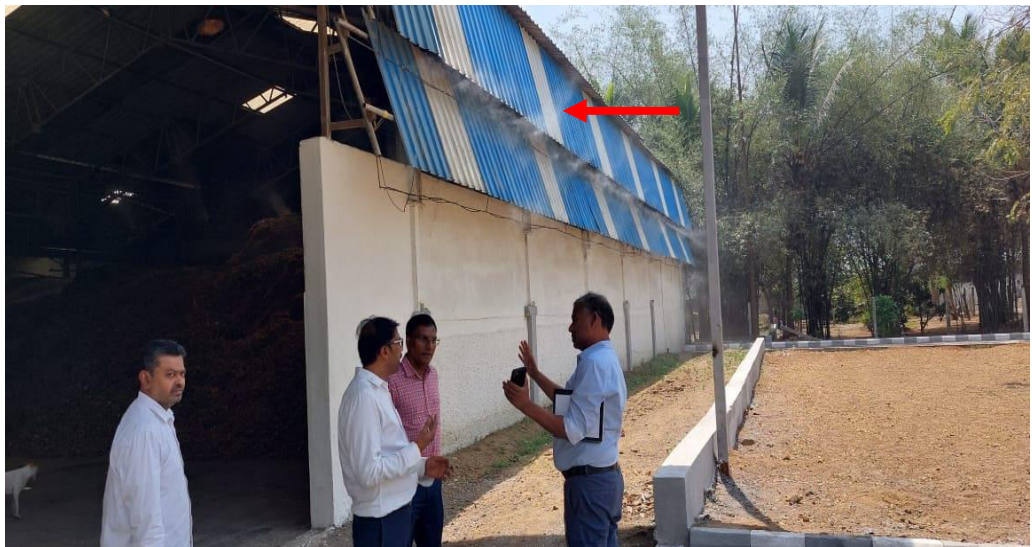
Mist filtration provided at Industrial louvers of unit shed
