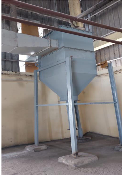
Gravity Ash collection box attached to Boiler
