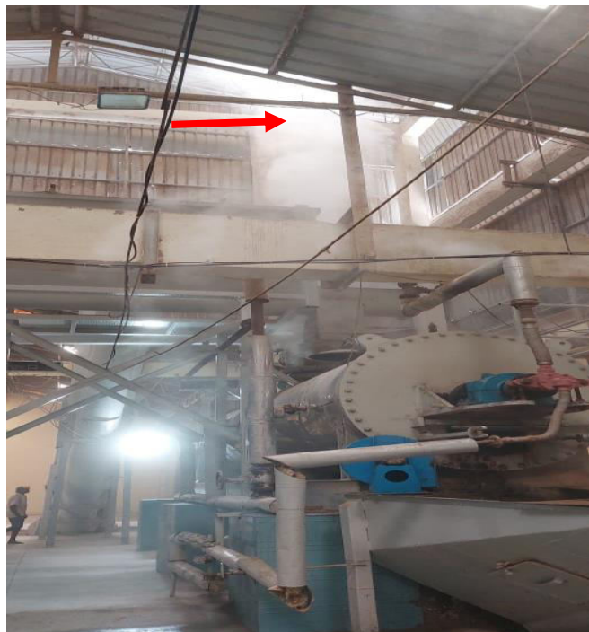
Odour containing vapour escaping from digester without any control measure
