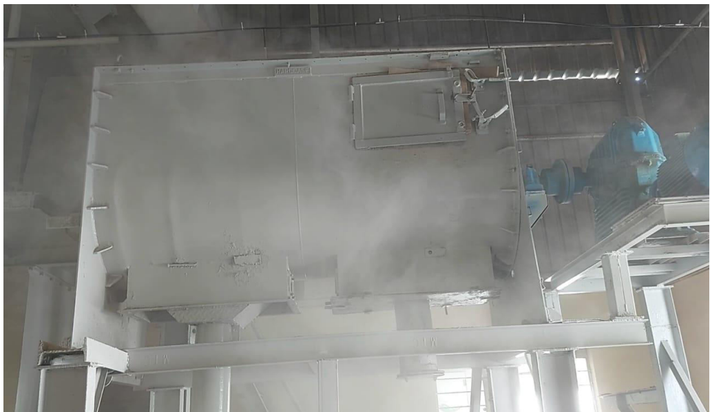
High Dust generation from pulverizer during operation
