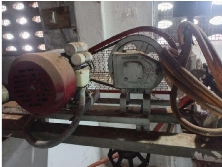
Water Jet arrangements & ETP
