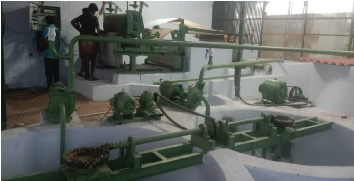
Paper pulp in settling tank
