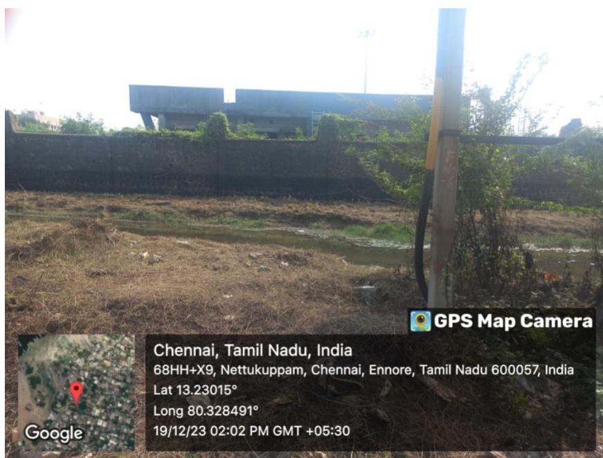
Photo showing oil spillage residues on compound wall near to the drain
