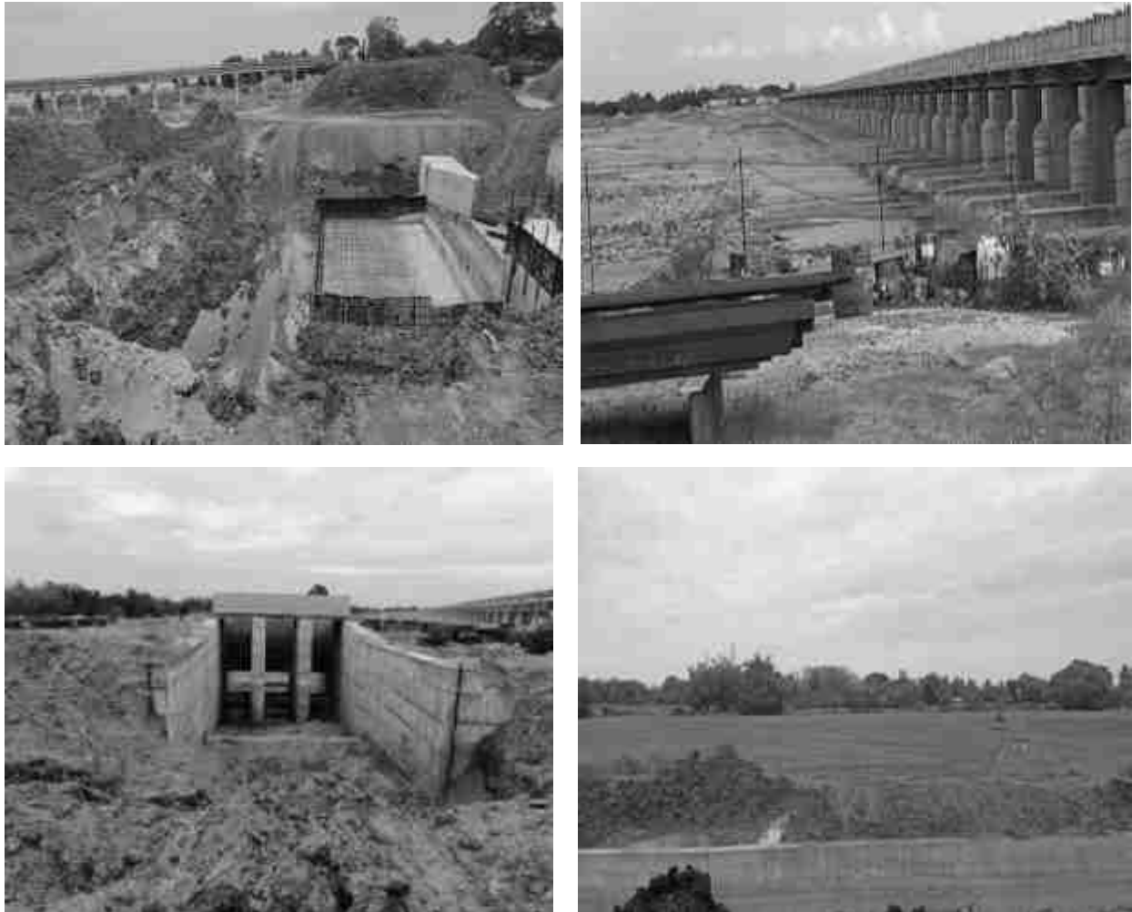
Fig 13.1 Showing improper dumping of earth and scattering of construction materials, wastes
